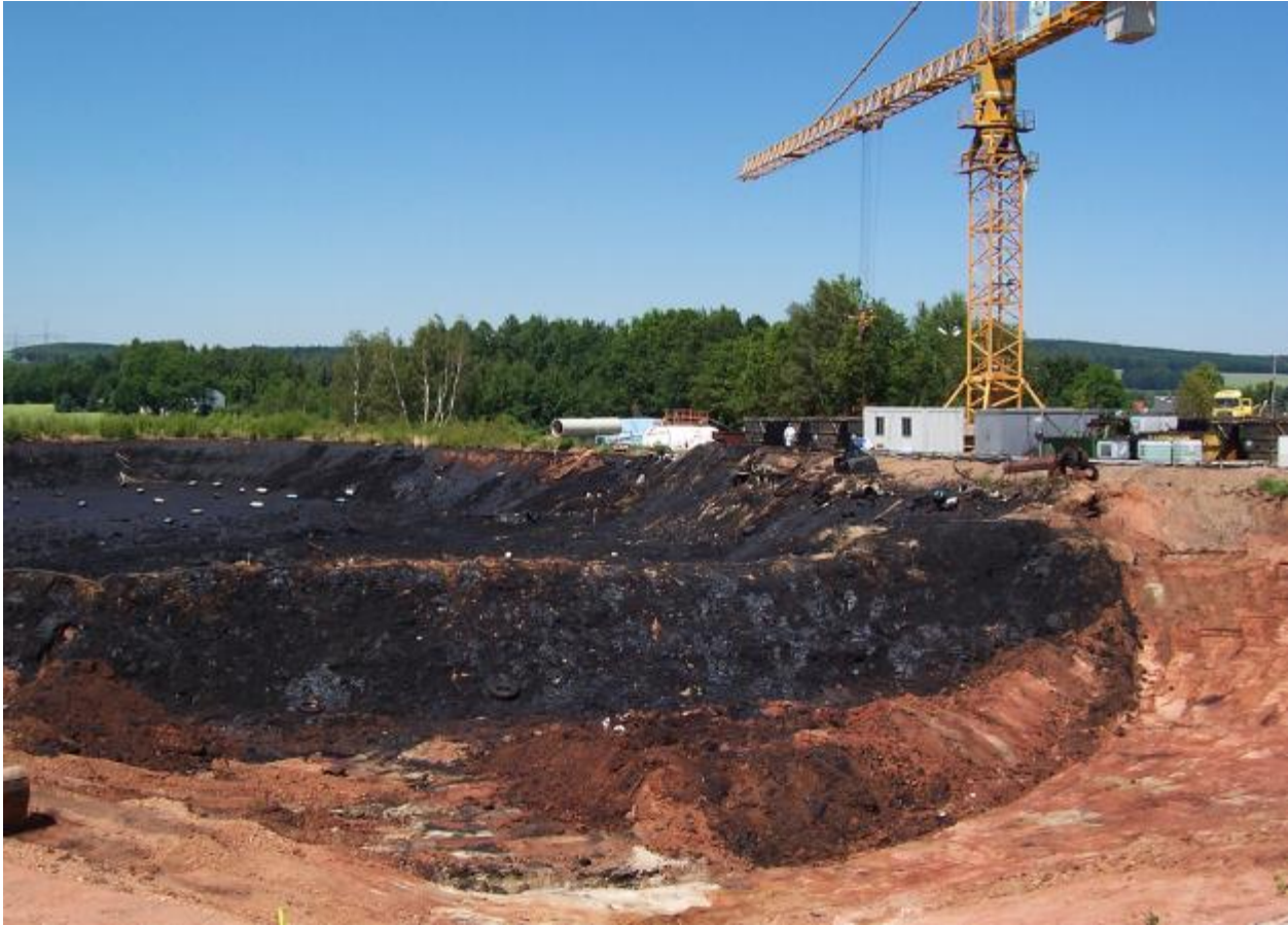
Figure 4: Excavation of the different parts of the acid tar lagoon in Mittelbach
