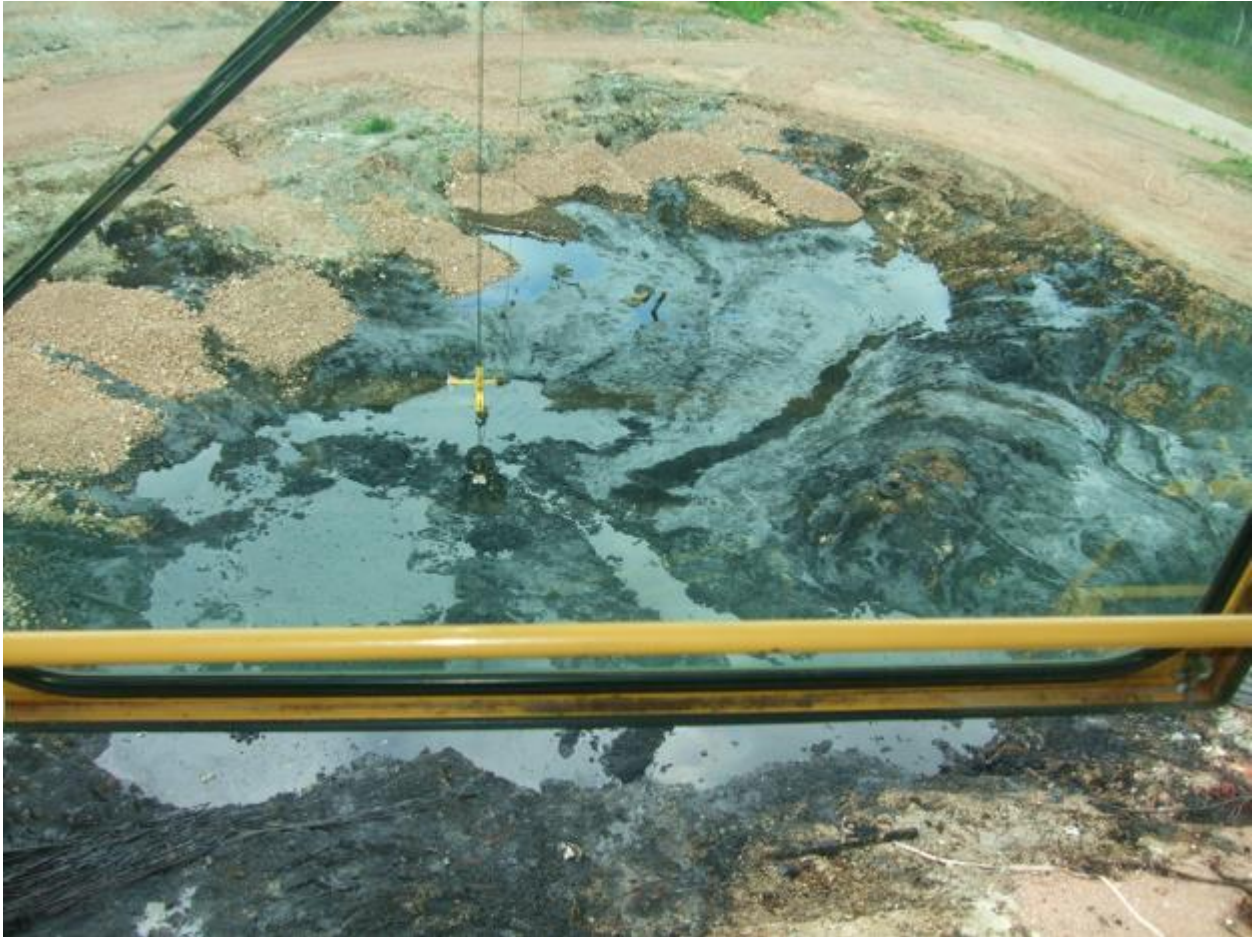
Figure 5: Excavation of acid tars at the lagoon 3 in Neukirchen with stabilisation of dams
